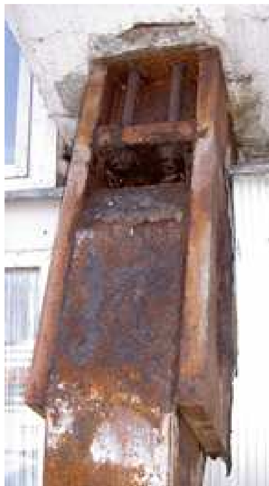
Fig. 4. The corroded joint of the tension rod.
