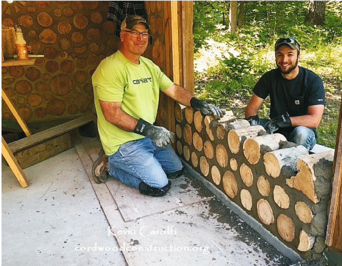
Fig. 2. This is the construction technique of cordwood masonry. Cordwood logs are placed in clay based mortar to build a wall; photo by: [Cordwood Construction, 2020]
