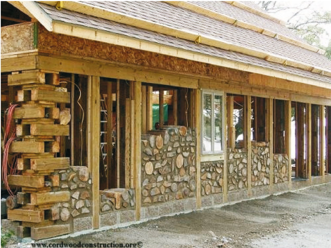
Fig. 18. An example of a load bearing frame with roof, and afterwards the work of making the cordwood wall; photo by: [Flatau, n.d.].
