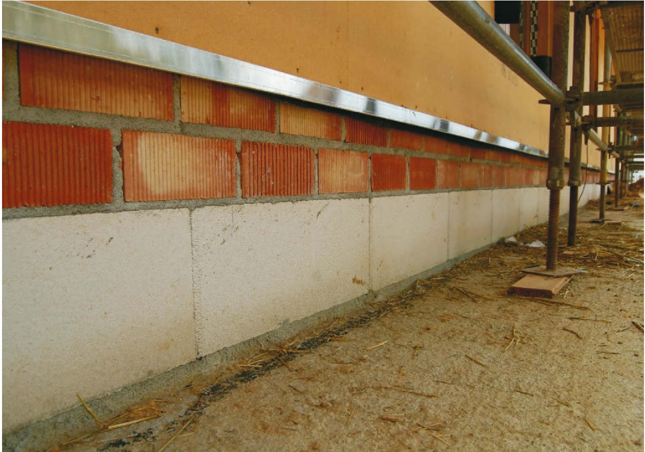
Fig. 43. The outside of a straw bale house, showing a sufficient height from the ground level of the sole of Portland cement. There is first a sole of Portland cement, then blocks and finally bricks. There is an impermeable membrane laid on top of the bricks, 2021; photo by the author
